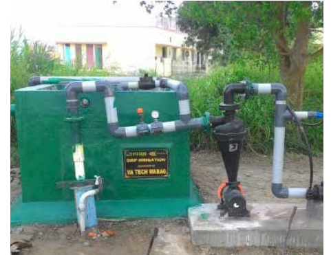
Right: Drip Irrigation System sponsored by VA Tech Wabag
